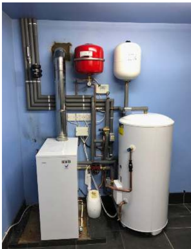
Tuscan 20/25 with 150 ltr. pressurised domestic hot water cylinder. (Replaced a combi boiler)
