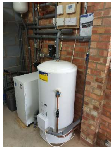
Tuscan 12/19 with 150 ltr. pressurised domestic hot water cylinder. (Replaced a combi boiler)
