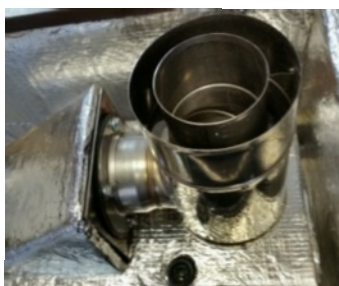
High level & vertical flue connection.
