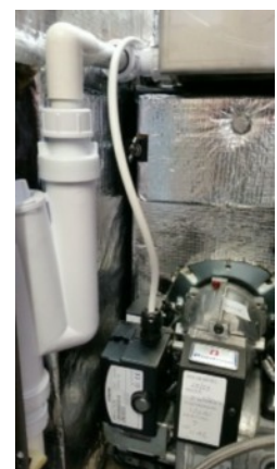
Condensate trap stays in situ for boiler service.
