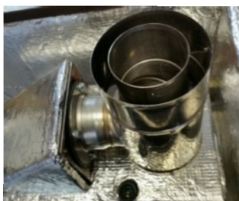
High level & vertical flue connection.
